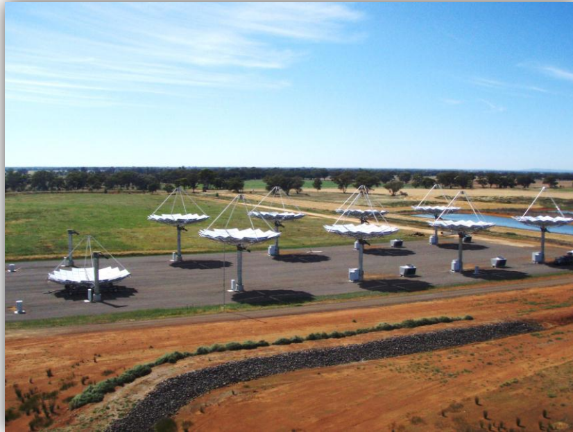
Recent photo of the Dish System Test Array under construction at the Bridgewater Demonstration Centre, Victoria
